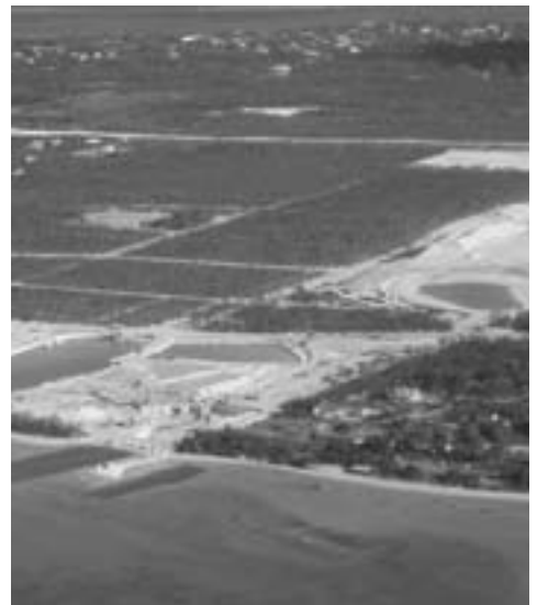
The construction of the Albany resort in the Bahamas is breaching the boundaries of the beach, allowing sea water to leach into the island's main fresh water supply.
